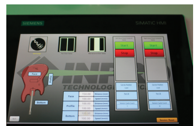
Figure 3. Operator HMI Screen on Chamber Controller. Image courtesy EIT LLC.
