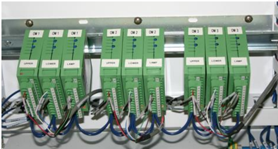
Figure 26: Multiple DIN Rail UV Intensity Monitors installed in a cabinet with different color wires used to identify individual Monitors
