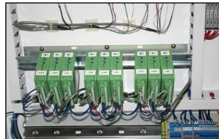
Figure 23: Multiple DIN Rail UV Intensity Monitors installed in a cabinet. Note labels on each DIN Rail to identify sensor location.
